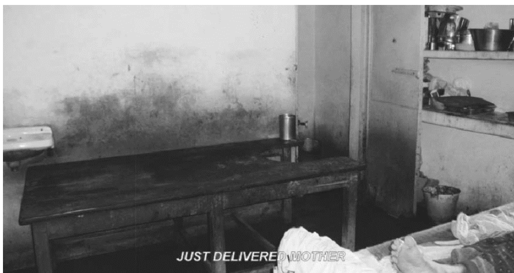
Figure 28: Sub-centre type A; with such unhygienic and inadequate delivery facilities pose a great risk to the mother and newborn (Indian Public Health Standards (IPHS), guidelines for sub-centres, Revised 2012)
